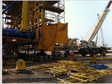
Production risers for offshore platform Northern Area Producing Division
