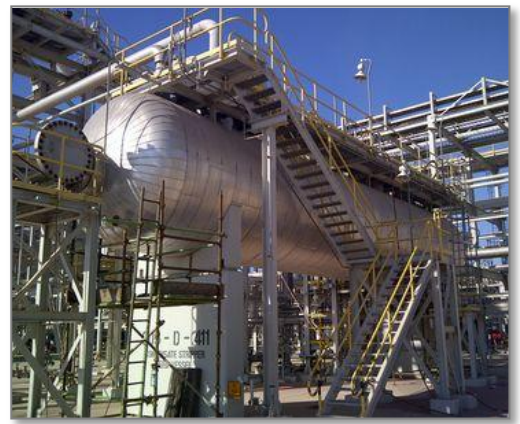
Condensate stripper Qatif – Gas and Oil separation plant #2
