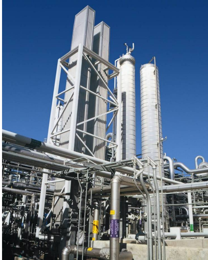
Zimpro wet air oxidation system for spent caustic treatment.
